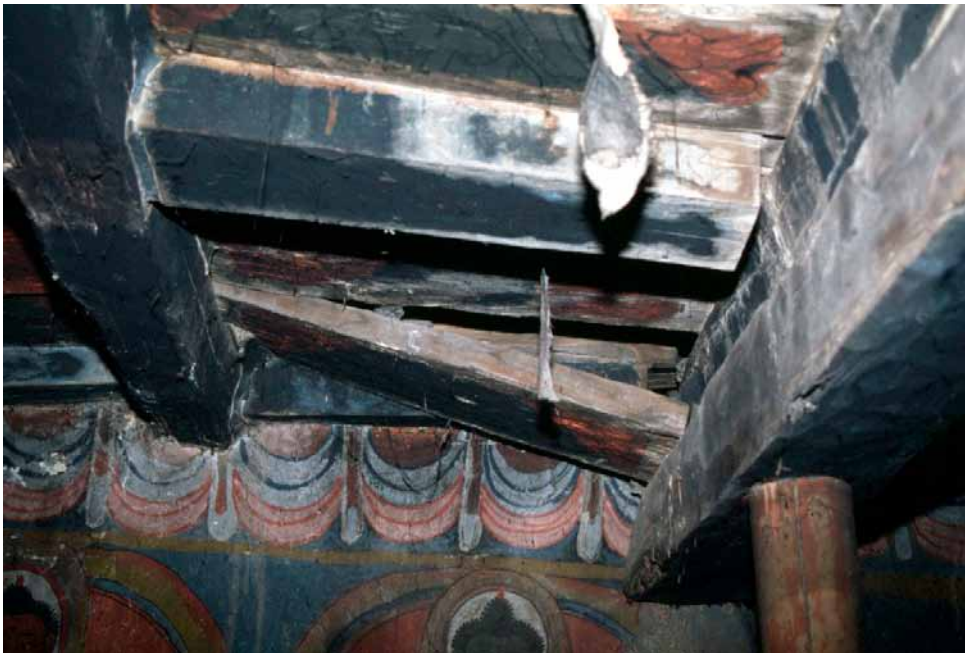
229 The red columns based on the gallery support the blue additional joists to secure the broken beams of the ceiling. They could be removed after the restoration work of the roof in 2008. HN 2004.
