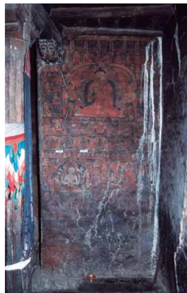
208 First floor north-western wall with water damage in the right corner. CL 2003.
