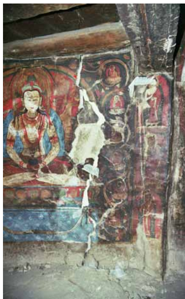
207 Second floor north-western wall with main crack in the main apse area. CL2003.
