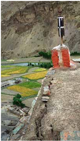
233 Crack on the eave caused by broken scantlings. HN 1998.
