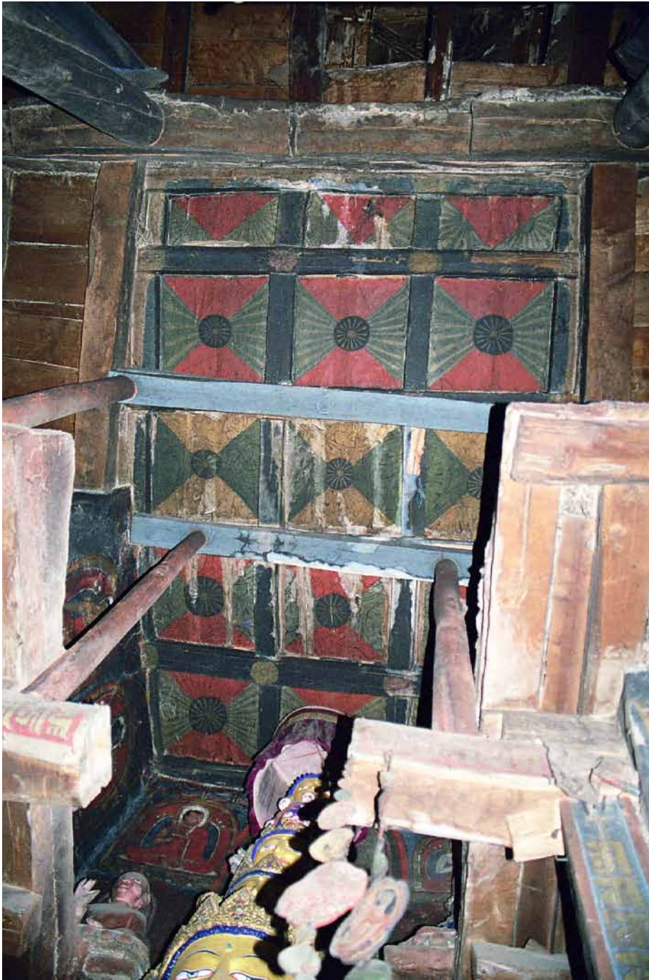
231 The false panelled ceiling over the main apse area. The substitutional construction for the broken beams were able to be removed in 2008. HN 2003
