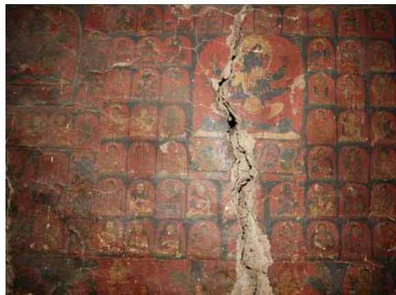
228 Crack of the south-western right side wall on the first floor. DL 2009.
