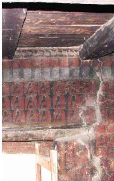
204 Main crack on the north-east wall of the second floor beside the entrance door. CA 2005.
