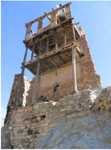
25 The wooden timber construction in front of the massive stone and brick walls. CA 2005.
