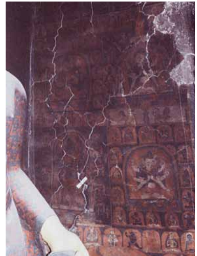
219 Crack on the right wall of the north-western niche. CL 2003.
