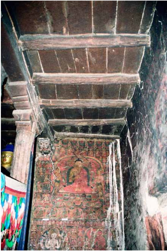
225 Murals damaged by water on the first floor in the right corner of the north-western wall. HN 2003
