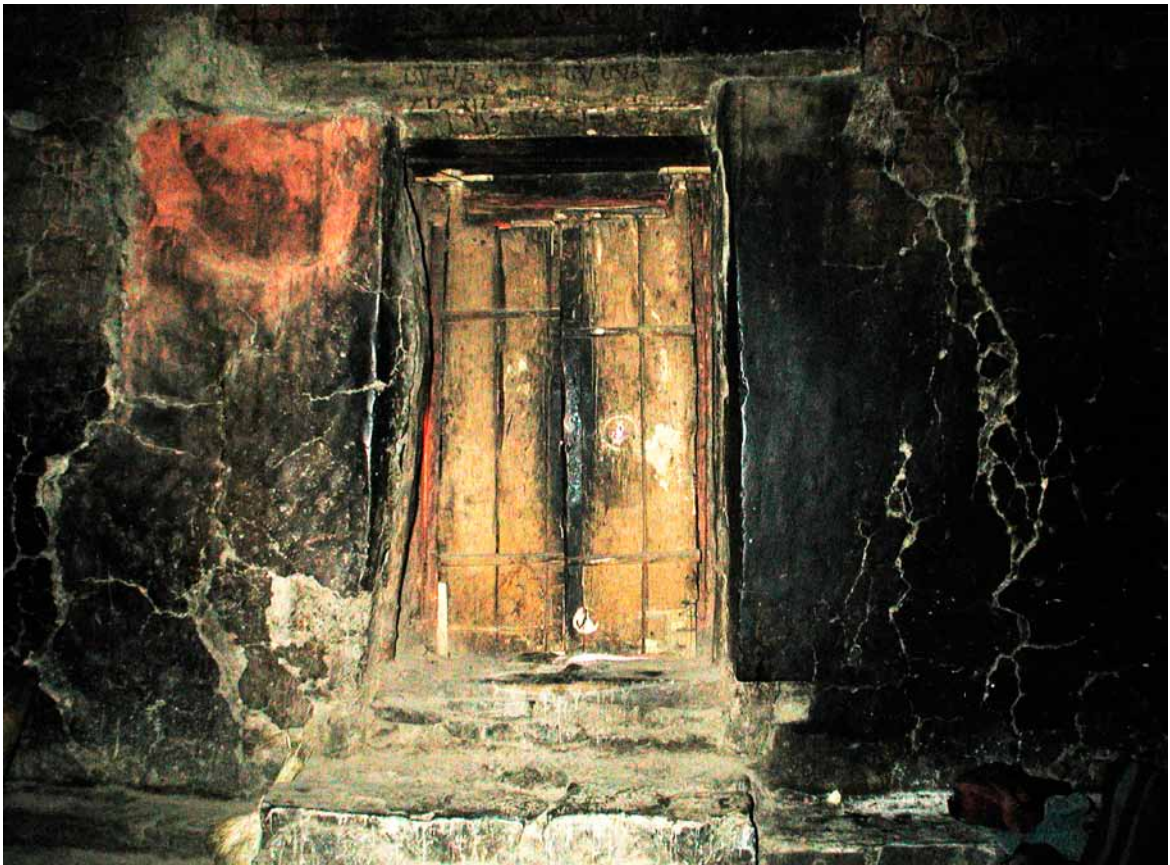
202 Entrance door on the ground floor of the the north-eastern wall. Between the main cracks and the left side of the door the paintings are completely destroyed. CL 2003.
