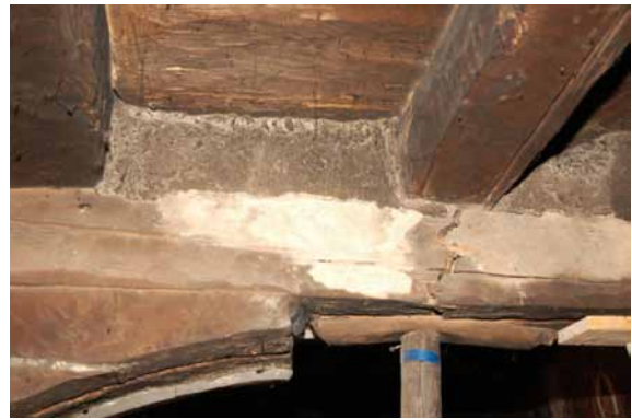
222 Detail of the broken main beam. DL 2009.
