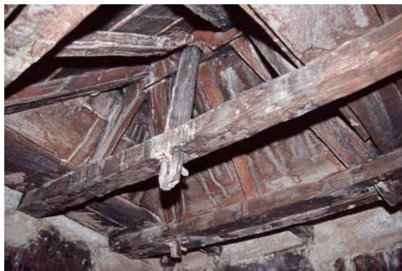
95 Details of rafters inside the hipped roof of the lantern. The pole holding the victory banner outside is fixed to the central beam with a wedge. CL 2003.
