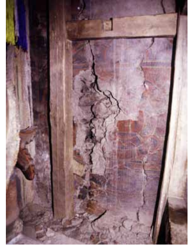
217 Settlement crack on the right wall of the main apse. CL 1998.
