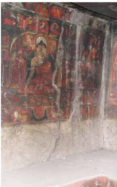
206 Main crack and water damage on the second floor of the south-eastern wall of the corner. CA 2005.
