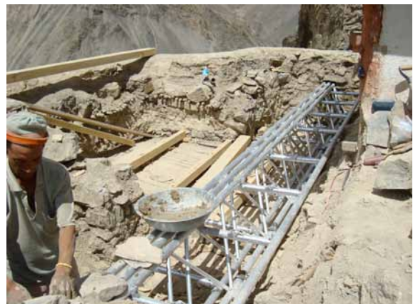
224 Assembling of the aluminium-lattice girder in place of the flat roof's broken wooden construction by the Achi association. Roland Pabel 2008
