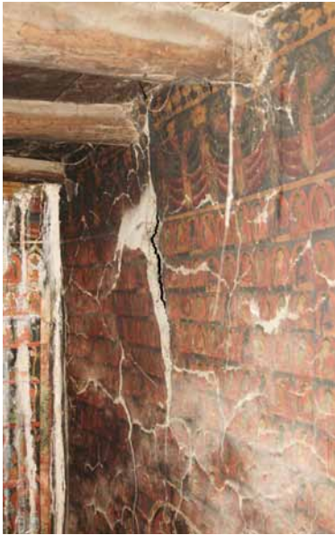
203 Water damage in the left corner of the first floor and the main crack on the north-east wall. DL 2009.
