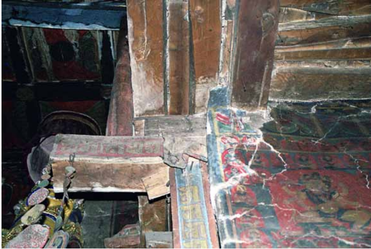
216 Right corner of the main apse below the gallery corbels with former repairs. HN 2003.
