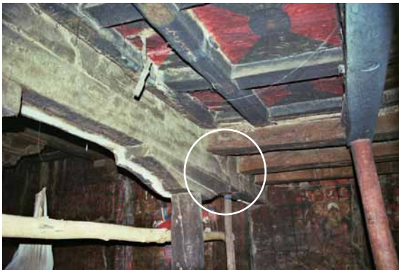
221 Location of the fracture on the back of the main beam. HN 2004.
