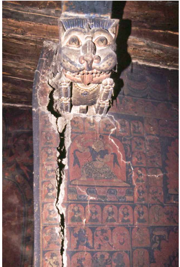
212 South-eastern niche with settlement crack beside the lion corbel. CL1998
