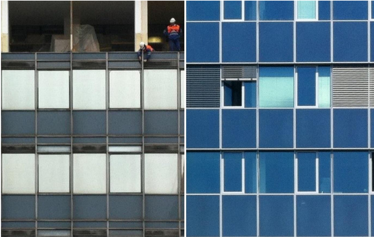
Figure 1: Retrofit of the campus building (2013). Left: dismantling of original curtain wall from 1971 (overall U-value approx. 3.0 \text{ W}/(\text{m}^2\text{K}) ). Right: New curtain wall, triple glazing, venetian blinds motor controlled, overall U-value 0.7 \text{ W}/(\text{m}^2\text{K}) by 60% glazed area
