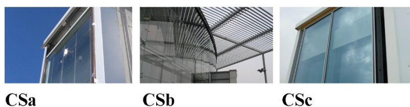
Figure 5: Monitored active transparent façades
