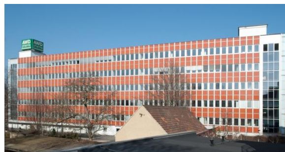
Figure 2: Type Leipzig, weather shell made of enameled single-pane safety glass, Radebeul Wasastraße.
