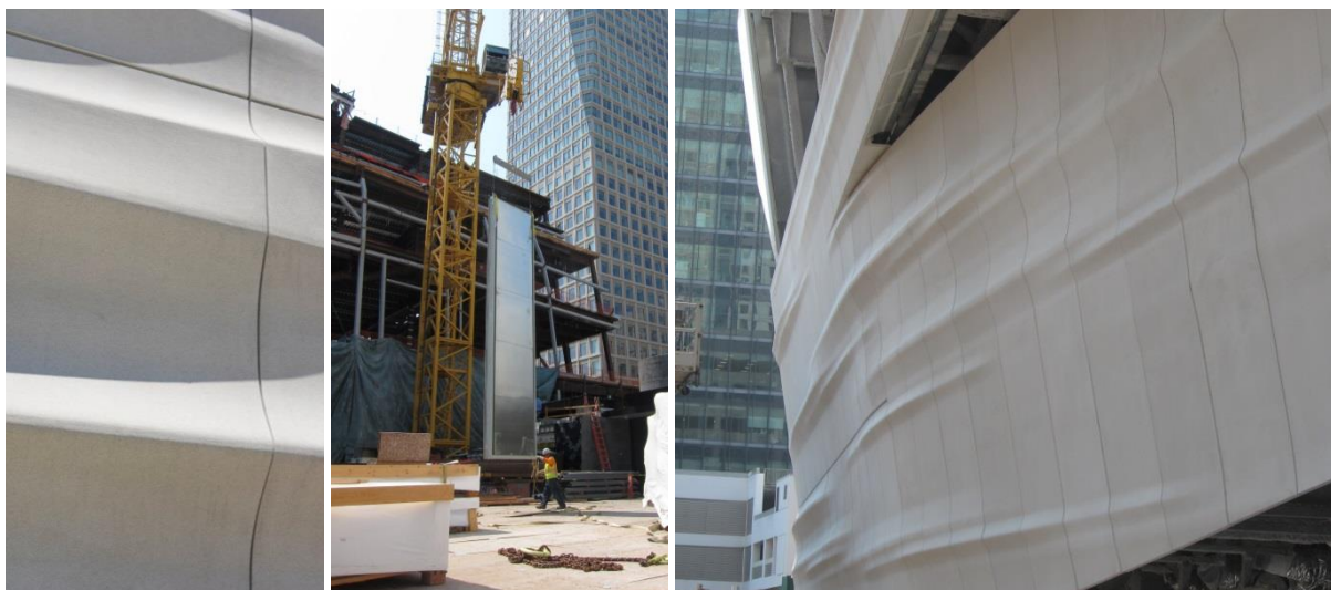
Figure 7: Photos from the enclosure installation at the project site: detail of contours and joints (left), unit size during rigging (middle) and continuity of ripples across units at lowest level (right).
