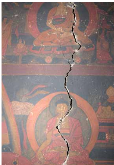
302 Cracks on the eastern wall. G&S 2011.
