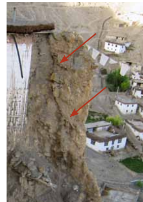
240 Detail of undermined kitchen foundation. K&S 2011.
