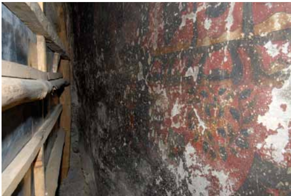
295 Western wall behind the wooden construction of the bookcase, fully covered with wallpaintings. G&S 2011 .
