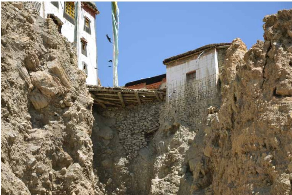
19 Terraces in front of the east facade of the main building. CA 2011.
