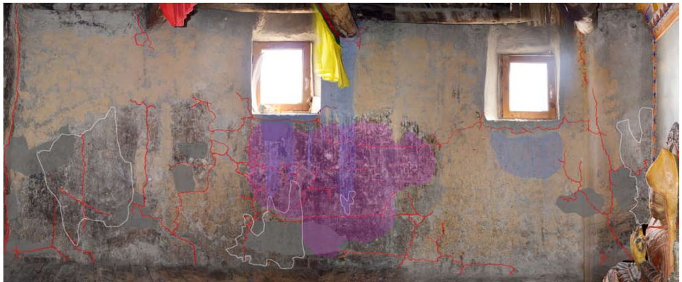
294 Map of the assembly hall. The southern wall showing voids, cracks, washouts and drips, flaking and thinned painted surfaces. University of Applied Arts Vienna 2011.
