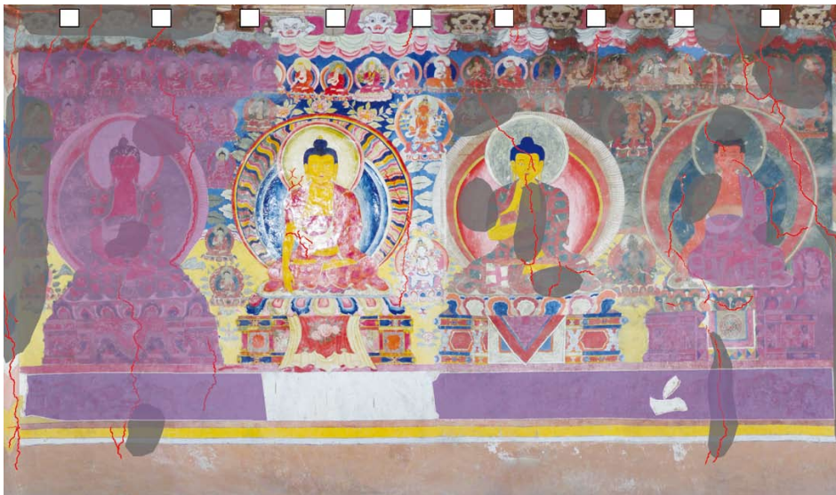
318 Map of the upper temple. The north-west wall showing voids, cracks, washouts and drips, flaking and thinned painted surfaces. University of Applied Arts Vienna 2011.
