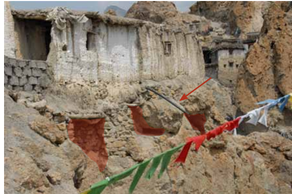
261 Underpin foundation elements along eastern side of the upper temple, and prevent water discharge over cliff. K&S 2011.
