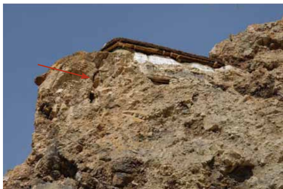
226 Tensile fracturing adjacent to monastery structures. K&S 2011.
