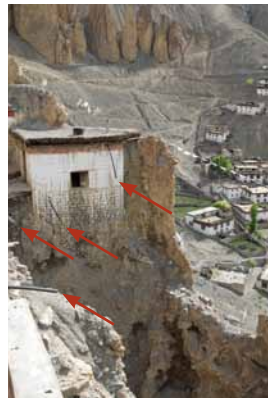
252 Prevent water discharge into gully along eastern side of the ancient monastery. K&S 2011.
