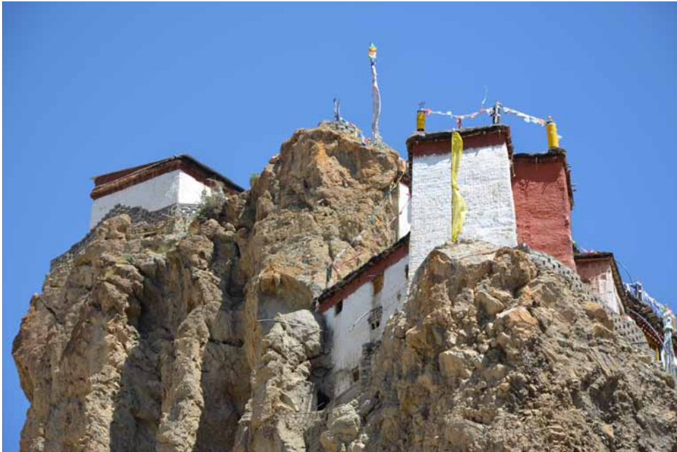
18 Retaining walls at the southern and western side of the monastic complex. CA 2011.
