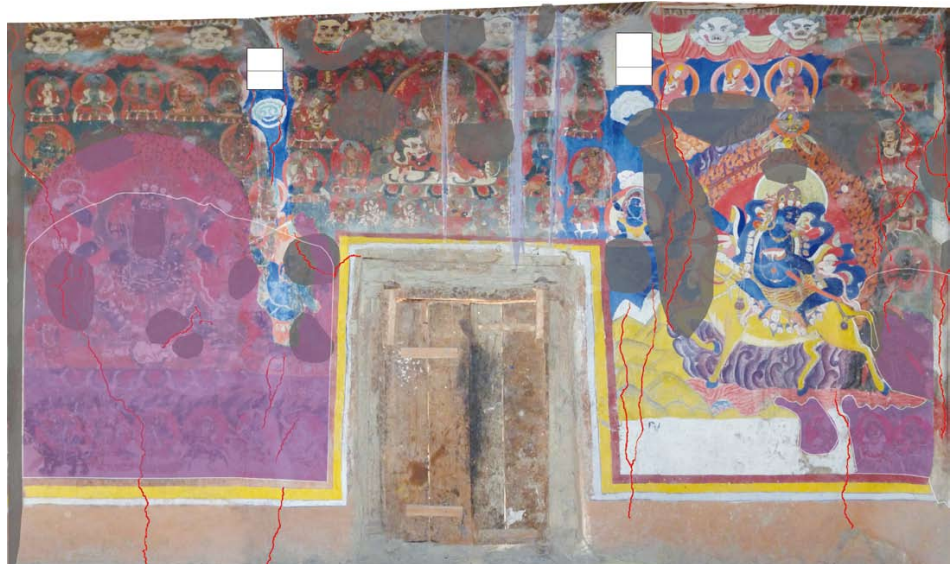
312 Map of the upper temple. The north-east wall showing voids, cracks, washouts and drips, flaking and thinned painted surfaces. University of Applied Arts Vienna 2011.
