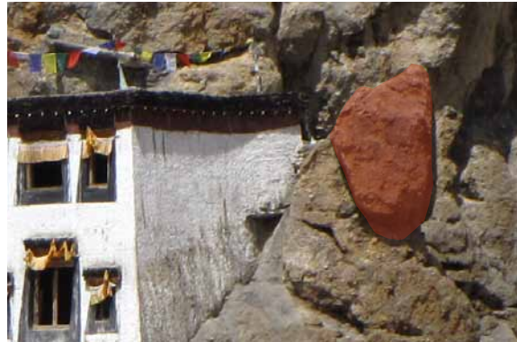
259 Potentially unstable block along northern side of the tower. LN 2011.
