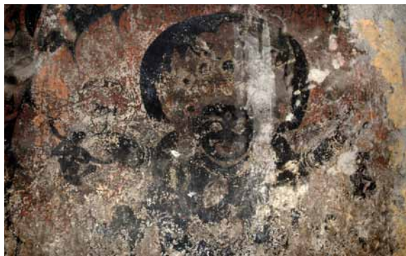
300 Wallpainting next to the entrance. Flaking areas and losses of paint layers. G&S 2011.
