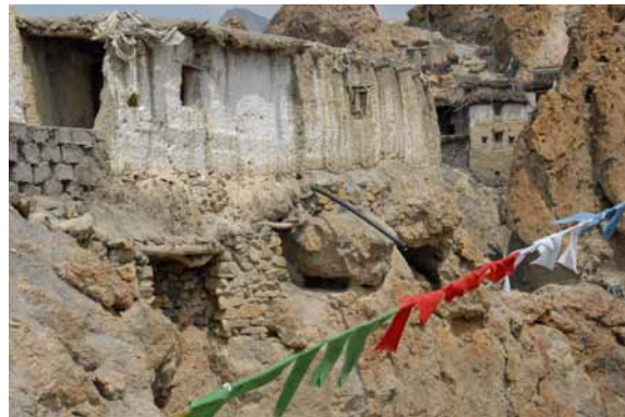
247 Foundation undermining along eastern side of the upper temple (note block and mortar underpinning, spanning timber beams and drainage pipe). K&S 2011.
