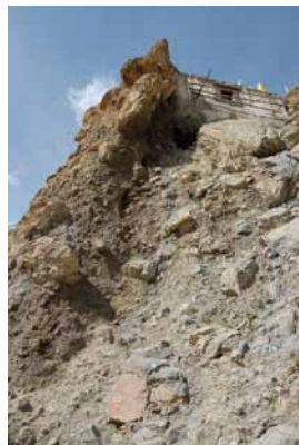
238 Tensile fracturing of bimrock fin along eastern side of the kitchen. K&S 2011.
