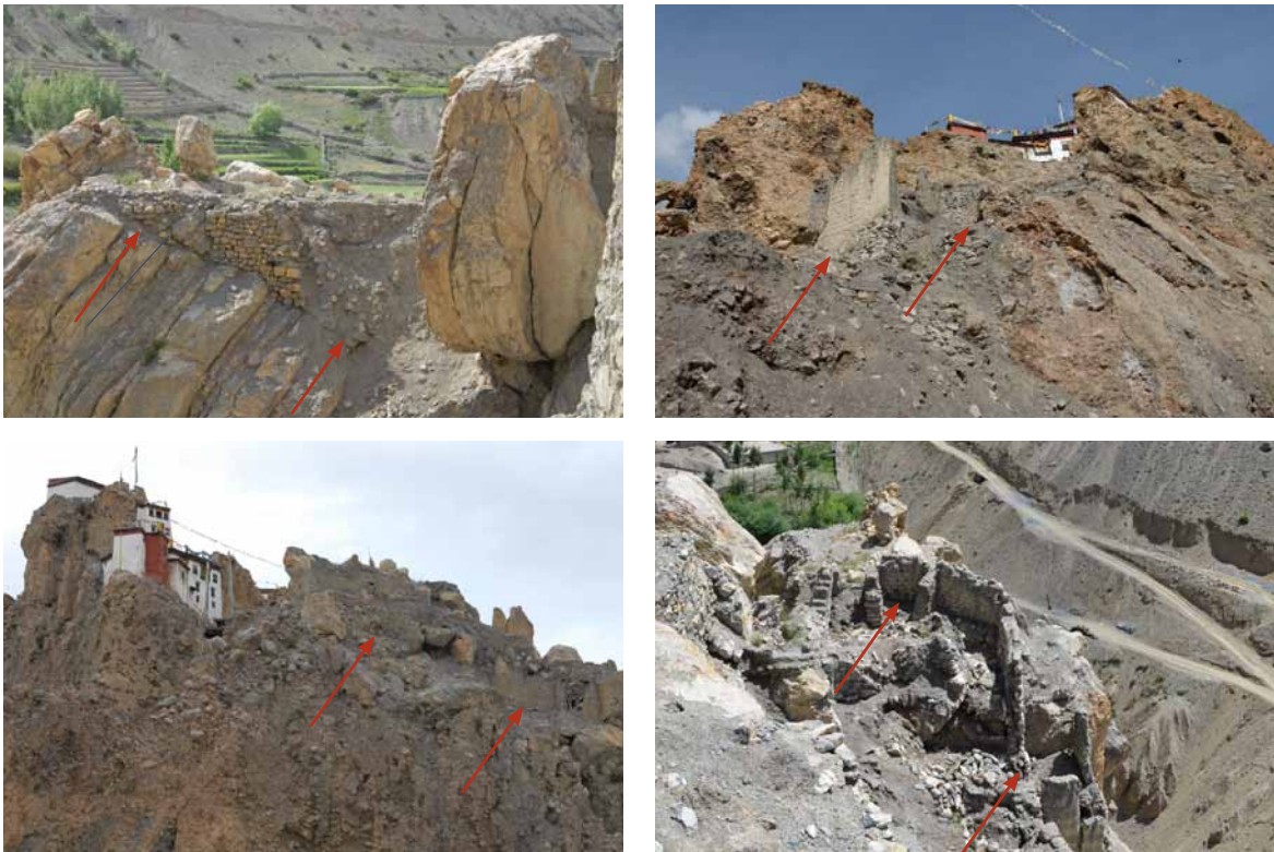
207 Foundation remnants within areas 1 and 2 of figure 206 (arrows point to the foundation - earth interface). K&S 2011.
