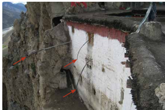
255 Prevent water discharge over southern supporting cliff of the ancient monastery. DB 2010.
