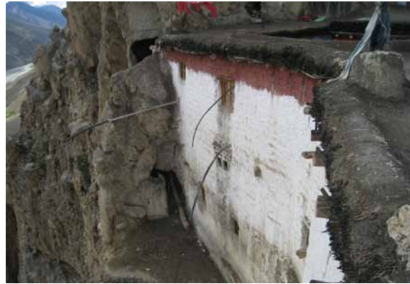
235 Drainage pipes at the southern facade of the monastery. CA 2011.
