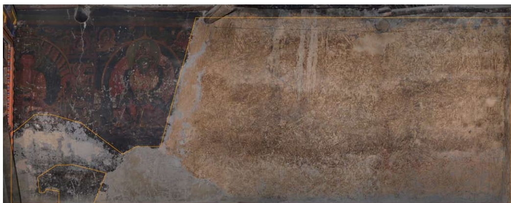
289 Map of the assembly hall. Northern wall with the extent of undecorated plaster, repair and recoated surfaces indicated. University of Applied Arts Vienna 2011.
