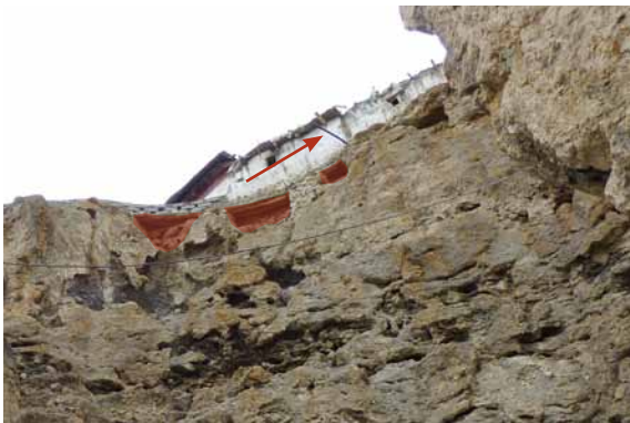
262 Underpin foundation elements along eastern side of the upper temple, and prevent water discharge over cliff, seen from below. K&S 2011.
