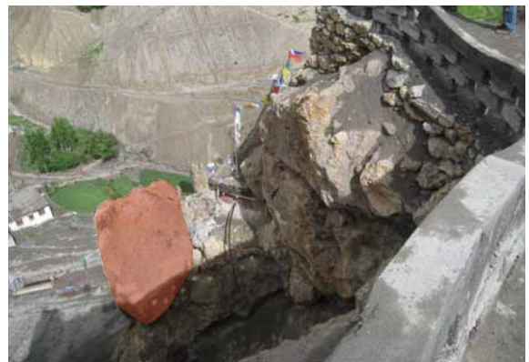
243 Potentially unstable rock block adjacent to northern side of the tower. LN 2011.
