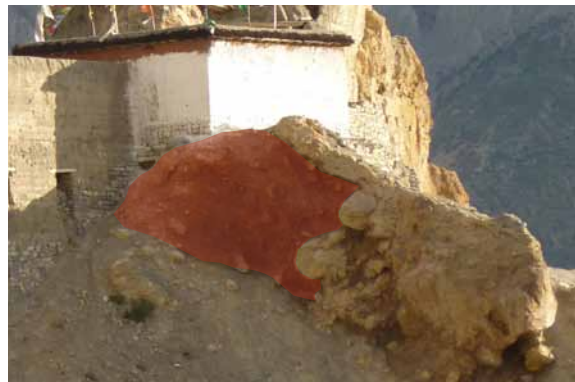
263 Overhanging slope at the castle of the No no. HN 2011.
