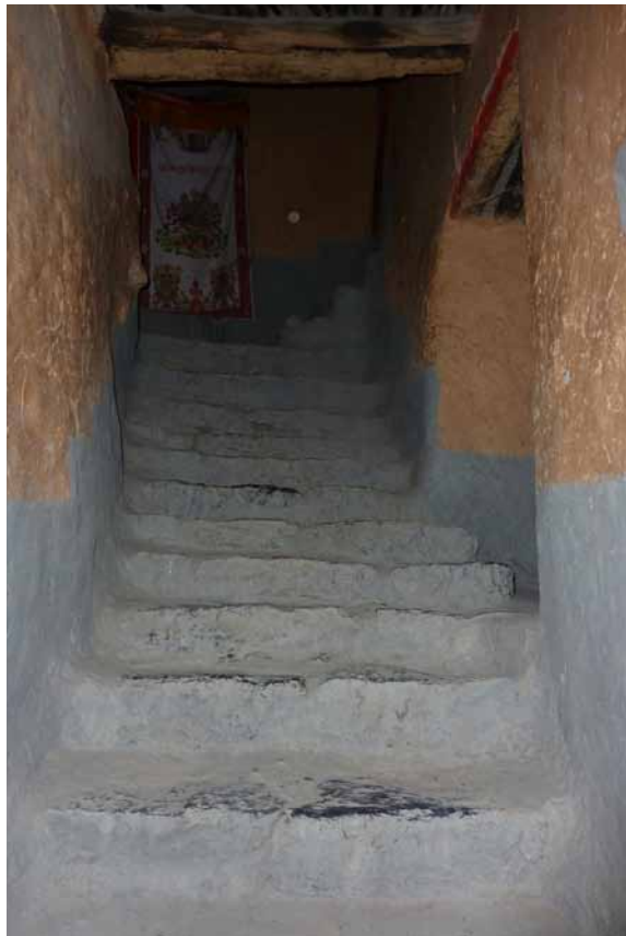
43 On the right the access to the anteroom of the assembly hall. HN 2010.
