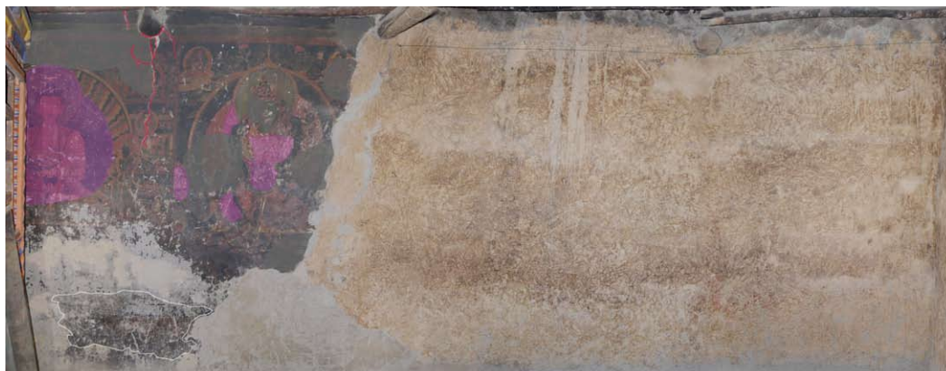
290 Map of the assembly hall. Northern wall showing voids, cracks, flaking and thinned painted surfaces. University of Applied Arts Vienna 2011.
