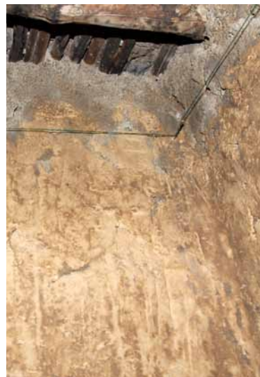
307 Unpainted surface in the north-eastern corner. G&S 2011.
