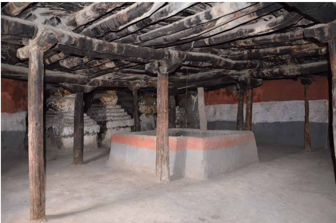
73 Middle area of the intermediate storey above the assembly hall with the parapet of the lantern. CA 2011.
