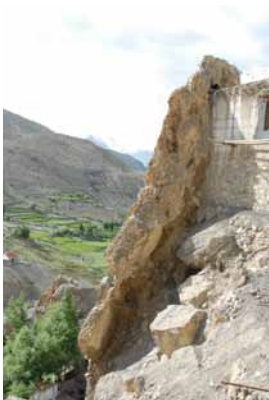
237 Erosion rill and partial undermining of foundation along northern side of the museum (note bimrock fin along eastern side). K&S 2011.
