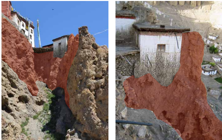
250 Shotcrete protection along eastern side of the ancient monastery and southern side of the kitchen. K&S 2011.
