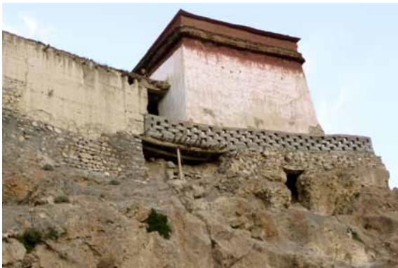
246 Foundation undermining along western side of the upper temple (note wood post and beams). CA 2011.
