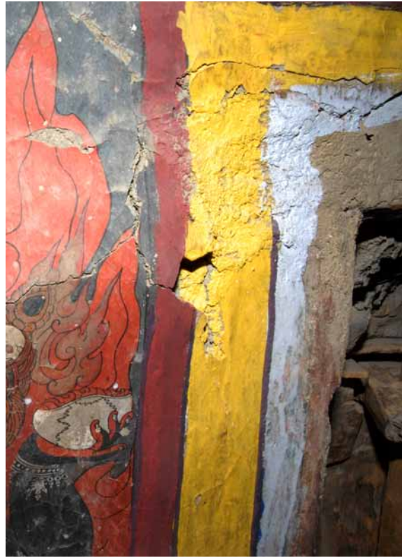
328 Voids, cracks and losses. G&S 2011.
