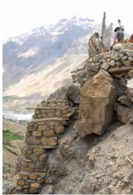
234 Partially undermined large block along eastern side of the ancient monastery. K&S 2011.
