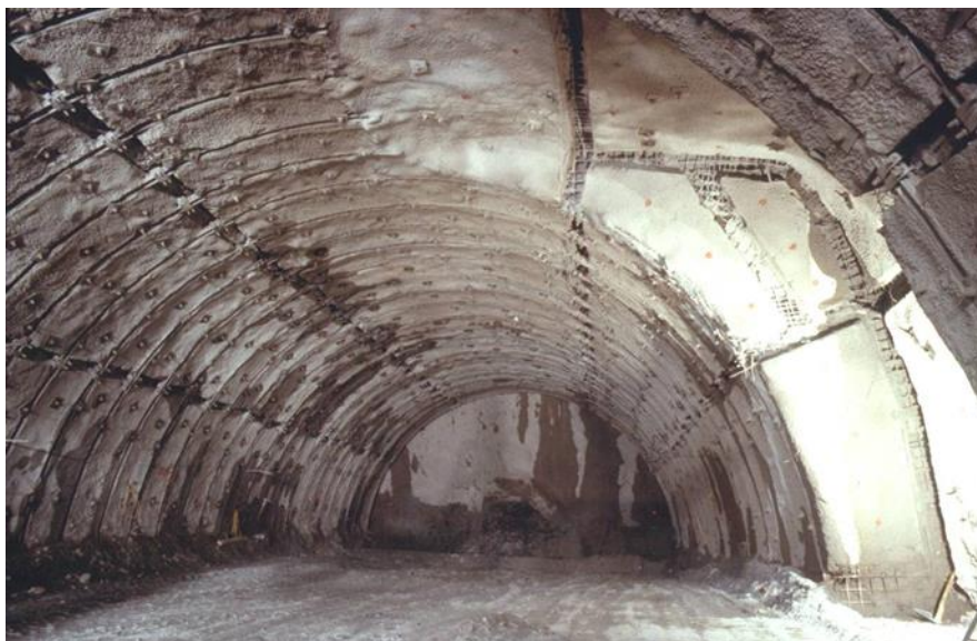
Figure 2. Open gaps in the shotcrete lining at the Inntaltunnel, Austria. Photo: Schubert
