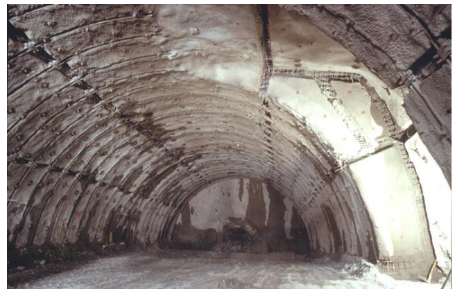
Figure 2. Support with open slots in the lining (Innatltunnel, Austria)
