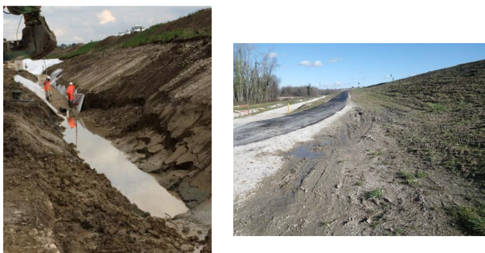
Figure 4: Picture of the draining ditch being excavated during works in 2014 (left picture), observation of humid soil (right picture).
