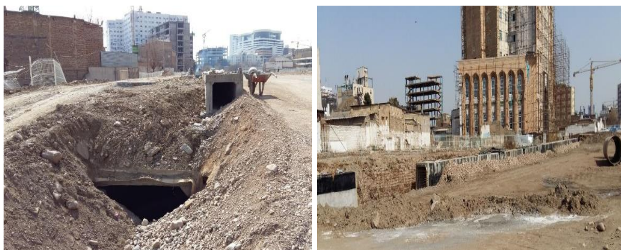
Figure 4. Energy tunnel in the distressed area of Mashhad city.
