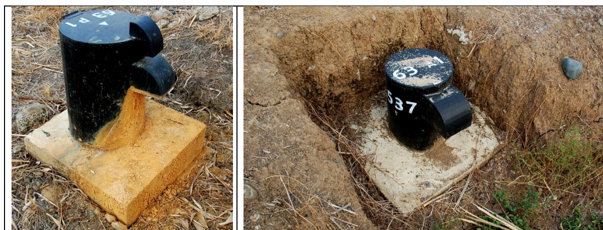
Figure 10: Daule Peripa reservoir rim dike, relief wells showing erosion and settlement cracks.
