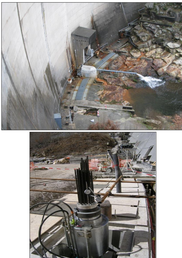
Figure 6 view of the downstream beam and of the installation of the anchors.
