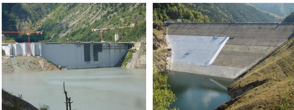
Figure 2. At left, PVC geocomposite sheets under installation on drainage geonet (the black material on top of the tendons and carbon bands mesh used for structural reinforcement) at Chambon dam in France in 2014. At right, PVC geocomposite sheets under installation on anti-puncture geotextile (the white material) in stage 2 at Pecineagu CFRD in Romania in 2012
