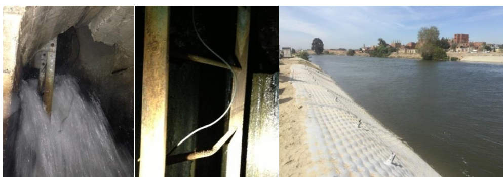
Figure 5. From left to right, joint 4-5 at Olai dam before and after underwater installation of Carpi external waterstop, and SIBELONMAT ® installed underwater at Ismailia canal, Egypt 2016
