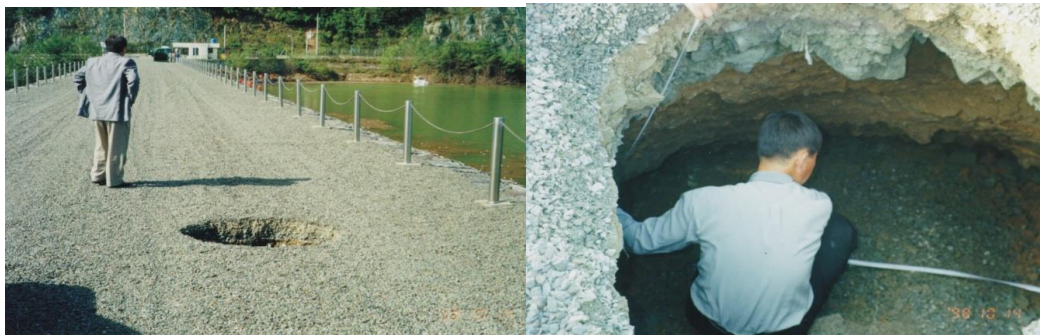
Figure 5. A sinkhole as a consequence of ageing that developed on the crest of the Unmun dam in 1998
