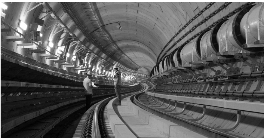
Fig. 10: Finished Metro Tunnel including Track
