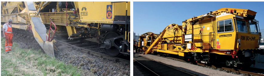
Figure 10: Excavating process on the construction site (left [51]) and ballast cleaning machine RM 80 UHR (right [52]).
