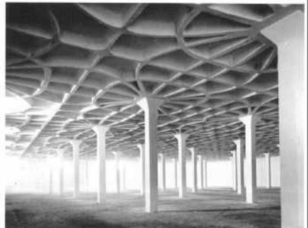
Lower level whose ribbed concrete slab optimizes material use and structural performance through the expression of the isostatic curves.
