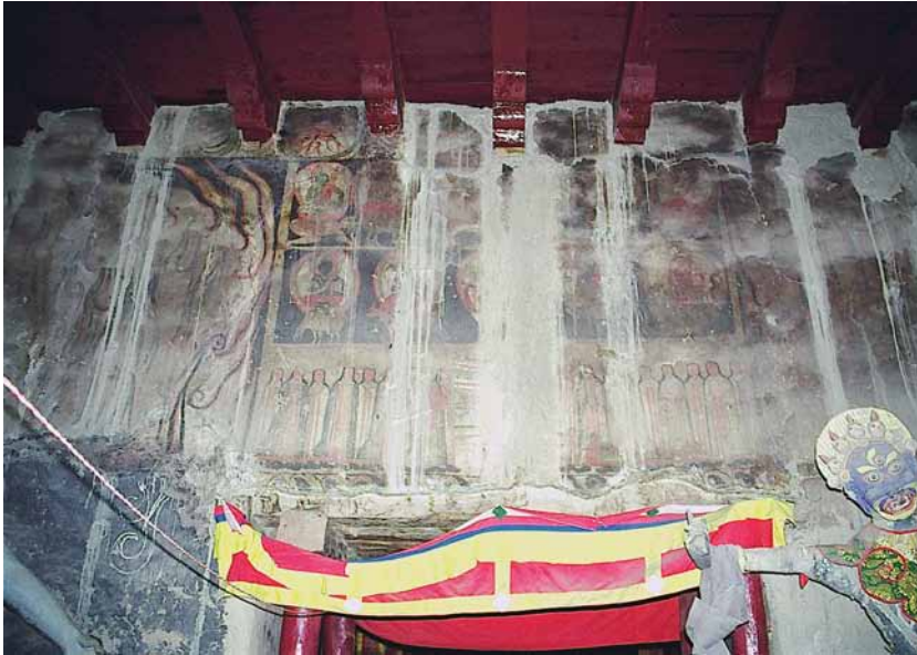
Fig. 245 Wall painting above the entrance to the assembly hall of the Main Temple. The traces of clay on the wall surface are due to water penetrating into the ceiling area, which affected the murals. Neuwirth 2002.
