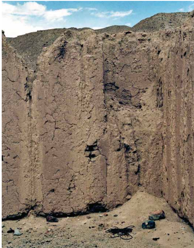
Fig. 466 Today, the north side room can only be accessed from outside through a small irregular opening on the west side. A construction seam next to the northeast corner of the main room could indicate the original access point. Neuwirth 2004.
