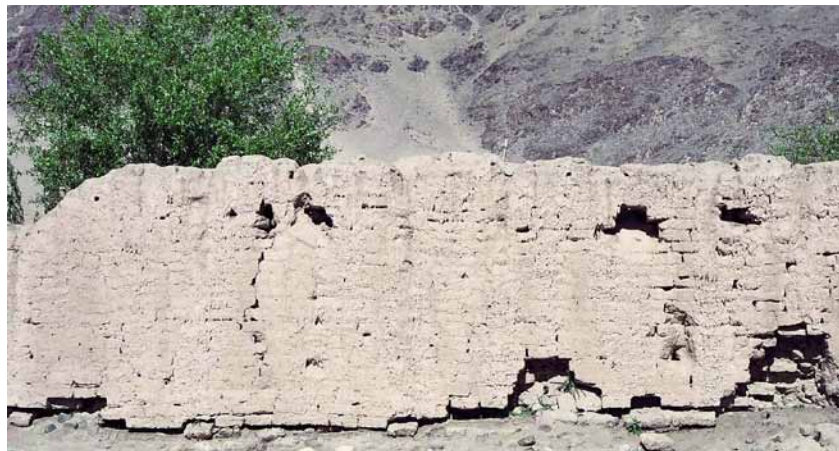
Fig. 490 The construction of the southern part of Nyarma's surrounding wall. The preserved fragments of Nyarma's boundary wall consist of a carefully assembled, originally plastered clay brickwork. Neuwirth 2003.
