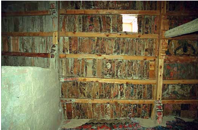
Fig. 382 The ceiling above the south wall of the Small 'Brom-ston Temple. The renewed areas are clearly visible on the wooden beams. Neuwirth 2002.
