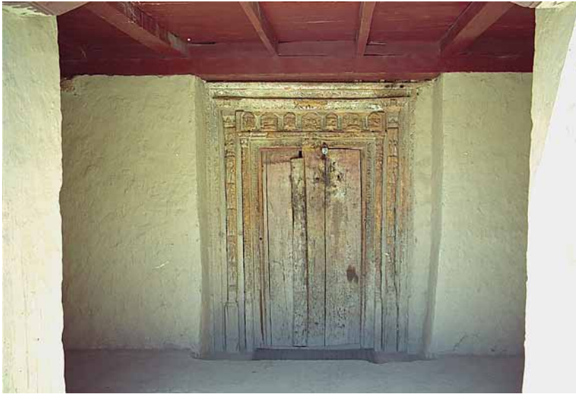
Fig. 403 The vestibule of the Maitreya Temple with the renewed ceiling construction and the entrance door to the temple interior. Neuwirth 2002.
