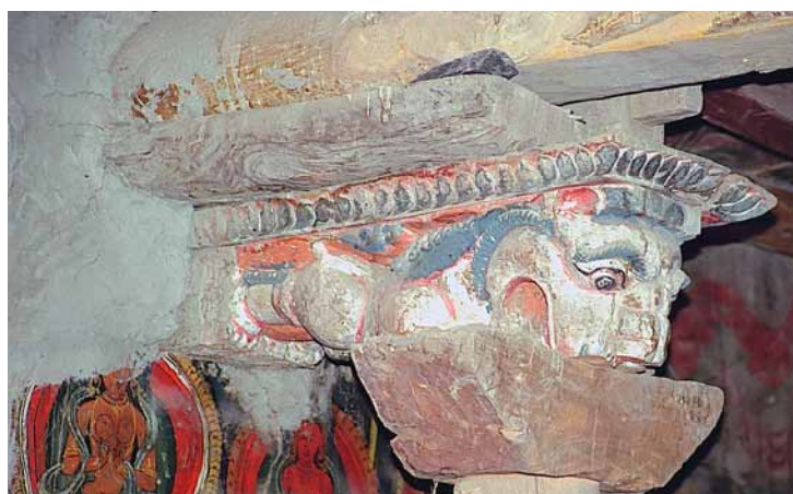
Fig. 313 The carved, coloured wall consoles, which are used as lateral supports of the main beams. The wall consoles were subsequently reinforced with wooden pillars. Above: the right console of the southern wall with the representation of a human hybrid. Middle: the left console of the north wall, showing another representation of a human hybrid. Below: the right console of the north wall, showing a representation of a lion. Neuwirth 2002.
