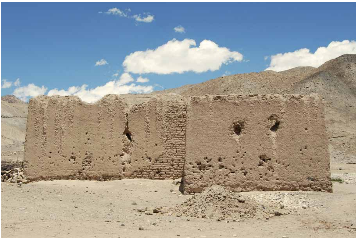
Fig. 459 The south façade of the temple ruin, showing the massive clay brick walls and parts of the plaster surfaces. Wrumnig 2012.
