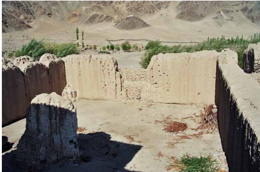
Fig. 165 View to the former entrance inside of the assembly hall, which has been bricked up. The remains of the throne-like bricked pedestal are located on the west side of the assembly hall. On the side walls of the assembly hall, the former position of the main beams can be identified along the upper edge. Auer 2003.
