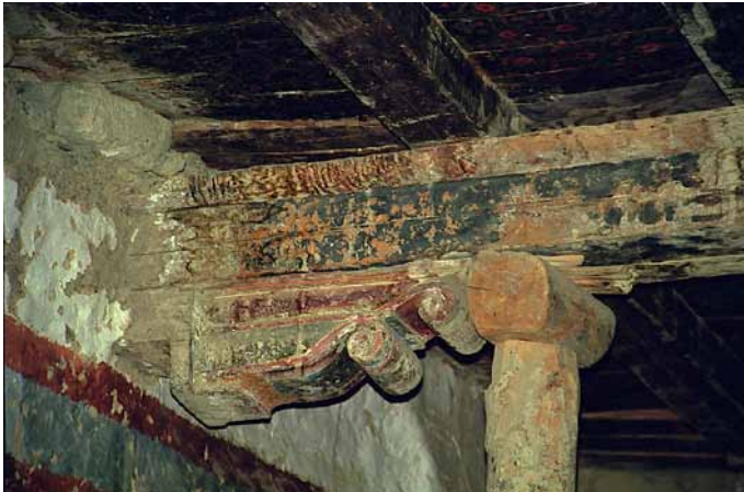
Fig. 414 Wall console of the main beam on the south wall with a support, which was installed later. Neuwirth 2002.
