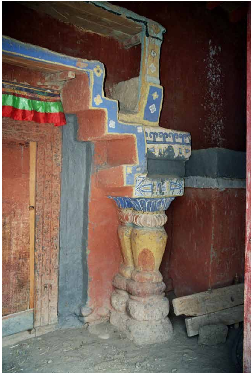
Fig. 113 Detail of the lateral structure around the plastically designed portal. Only fragments of the upper part of the portal are preserved. Neuwirth 2007.
