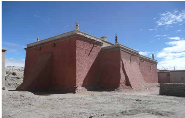
Fig. 585 The outer façades with supporting pillars at the Red Temple in Tholing, Auer 2007.
