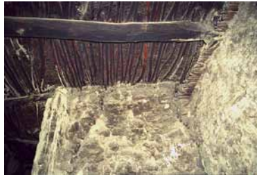
Fig. 276 Original eave details on the south outer façade of the entrance hall of the Main Temple, which have been preserved under the later erected ceiling construction. The picture on the right shows the corner on the façades between the vestibule and the assembly hall of the Main Temple, which today can be seen in the space in between. Neuwirth 2002.
