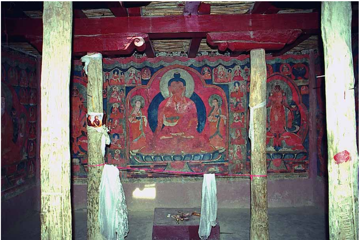
Fig. 365 The ceiling construction is supported by four simple wooden pillars. The capitals, main beams and secondary beams of the ceiling are painted red. In the background, the wall painting on the west wall is shown with the altar standing in front of it. Neuwirth 2002.
