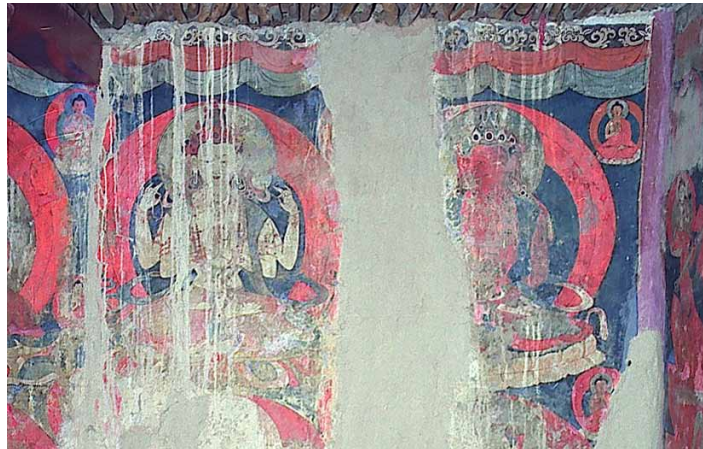
Fig. 589 White Temple of Tabo. Damage to the inner wall by condensation and the penetration of meteoric water. Neuwirth 2002.
