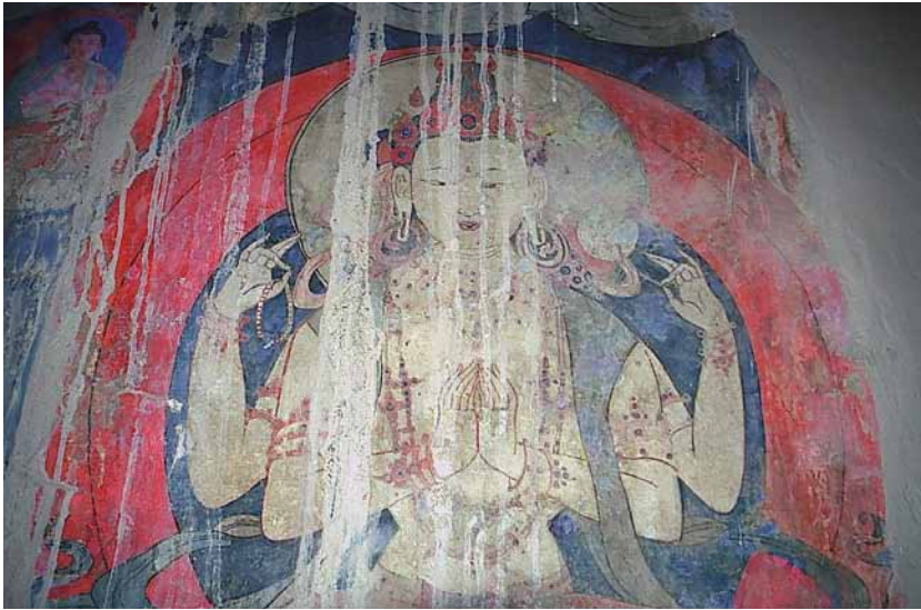
Fig. 364 Detail of the wall painting on the north wall with clear traces of water damage. Neuwirth 2002.
