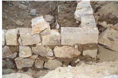
Fig. 554 Left: The course of the brickwork will be checked with a batter board, and the quarried stones will be straightened on the outside. Neuwirth 2002.
