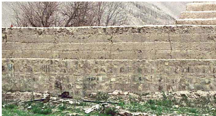
Fig. 491 The construction of the southwest corner of Tabo's surrounding wall after the renovation. The lower half consists of stone masonry; layers of rammed earth are clearly visible above this. Auer 2003.
