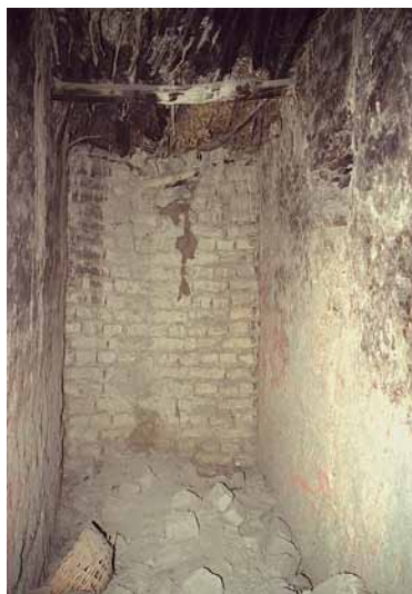
Fig. 278 The ceiling construction above the intermediate space consists of irregular round beams and logs. On the right, the west outer walling is visible, consisting of clay bricks which were not plastered inside. This walling closes the gap. Neuwirth 2002.
