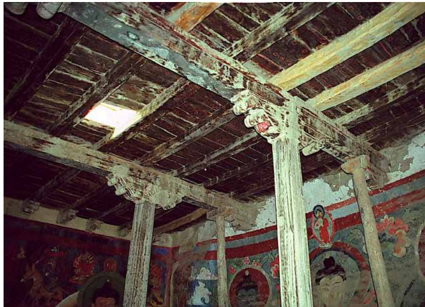
Fig. 413 View of the two main beams with the lateral wall consoles on the south wall. The second fracture in the plastered surface extends almost to the east corner; the repainting of the wall between both breaks is clearly distinguishable from the original wall painting by the colours and techniques used. The wall consoles of the main beams were reinforced by additional pillars. Neuwirth 2002.
