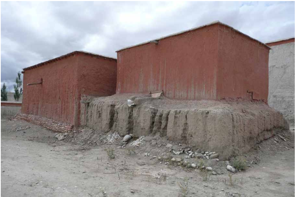
Fig. 68 Western view of the Golden Temple, with the preserved ground floor of the former three-storeyed structure. The façades of both temples have nearly the same height today. Auer 2007.
