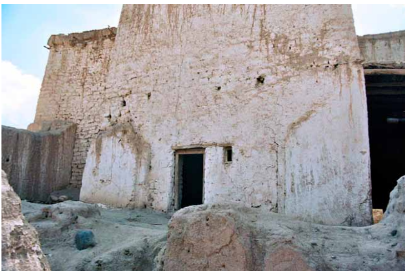
Fig. 168 The original wall opening of the cella was bricked up, but is still visible on the masonry around the current door. On its left, the inner ambulatory has been closed by a bricked wall to support the lateral rooms on the first floor. Auer 2003.
