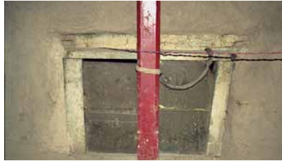
Fig. 272 Left: the west wall of the room above the New Entry Hall. Right: the hinged window on the north wall, which extends from the Protector Chapel below, into the upper floor of the New Entry Hall. Neuwirth 2002.
