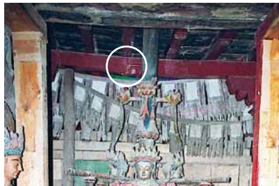
Fig. 569 Left: The crack in the middle of the wall at this ruin in Stok can be attributed to a weakness in the foundations as a settlement crack or it can be the result of an earthquake. Neuwirth 2000
