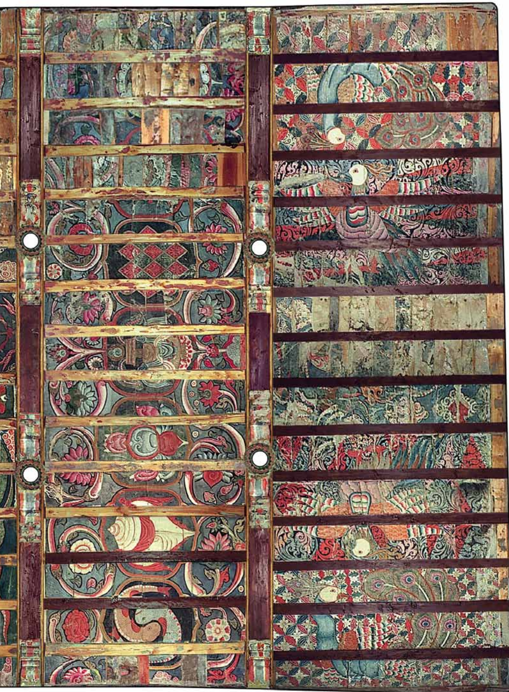
Fig. 290 Scaled photomontage of the painted wooden ceiling above the assembly hall and the apse of the Large 'Bromston Temple. Most of the fields of the wooden post ceiling are still painted, with the bays between the main beams painted with figures, animals, symbols and ornaments. © Neuwirth & Auer, TU Graz 2020.
