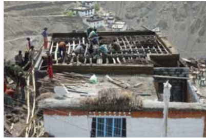
Fig. 572 Right: An insulating layer of grass and lichens is integrated into the first clay layer of the flat roof. Auer 2011.
