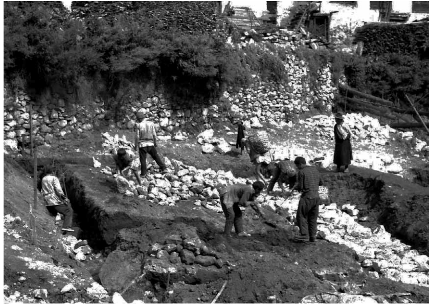
Fig. 560 Foundation work in Namche Bazar, a village in Kumbu at 3,440 metres above sea level. For the foundations, deep and wide trenches are dug, which are filled with quarried stones. Neuwirth 1975.
