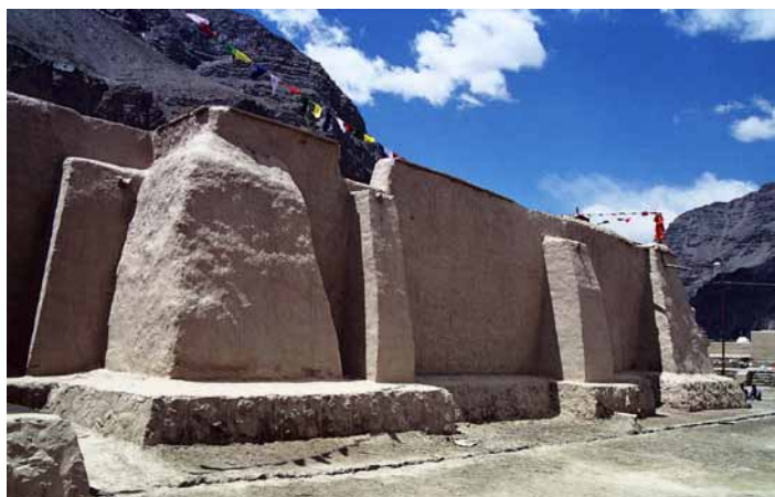
Fig. 587 Subsequently attached supporting pillars and a surrounding base zone on the north side of the Main Temple of Tabo, Neuwirth 2003.
