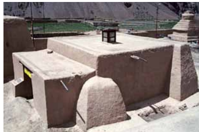
Fig. 577 Left: At the Mandala Temple of Tabo, the flat roof is still without attic in 2003. In 2019, the Mandala Temple has a raised parapet all around with the same number of water spouts without sufficient dimensions. Neuwirth 2003.
