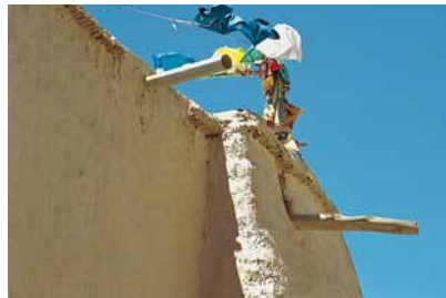
Fig. 575 Left: Water spouts of the Main Temple of Tabo. Beside the widely projecting wooden gutter, the dripping edge of the rod layer was removed when the new plastic pipe was moved. Neuwirth 2002.
