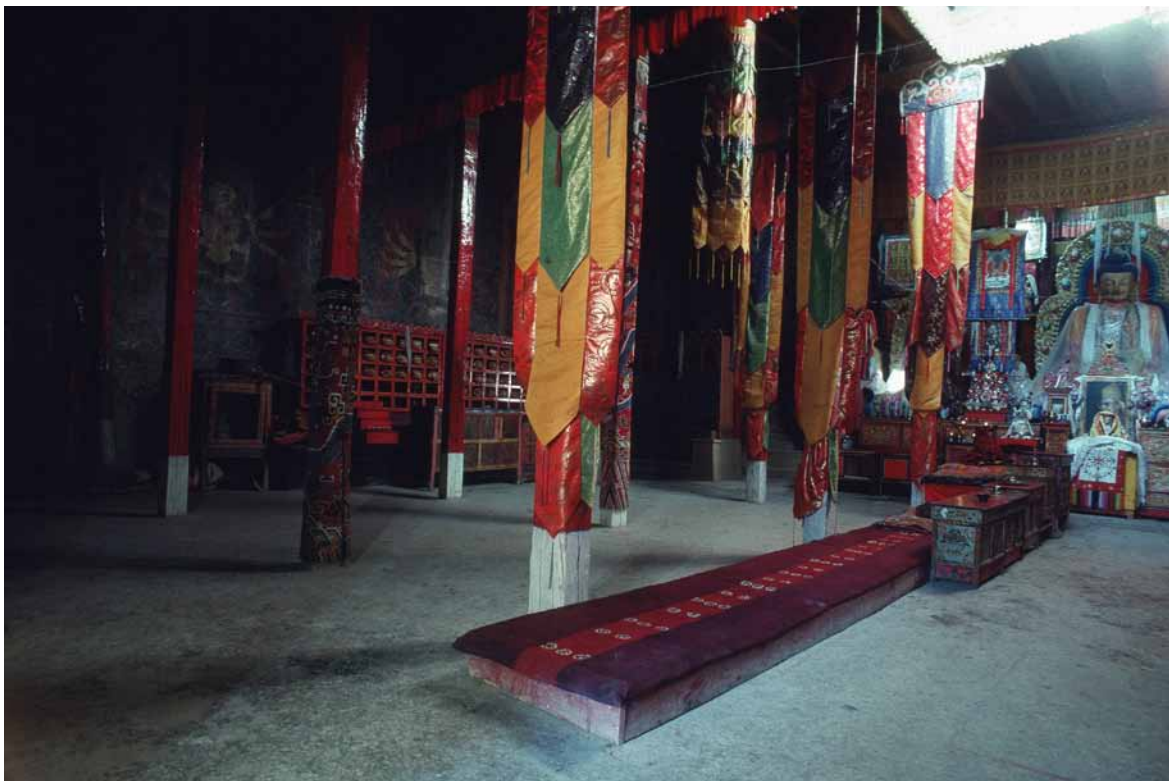
Fig. 101 The middle area of the assembly hall with the lantern in the ceiling. The wooden supports are spaced between 2.20 and 3.30 metres apart in a rectangular grid. The pillars and beams are painted red, and only the lower parts of the pillars are painted white. Poncar 1993, WHAV (JP93 45,02).
