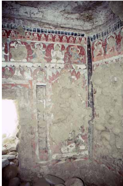
Fig. 209 The remaining murals on the northeast wall close to the low entrance-opening. The bearing stone elements of the roof construction are supported by painted stone corbels. Neuwirth 2003.
