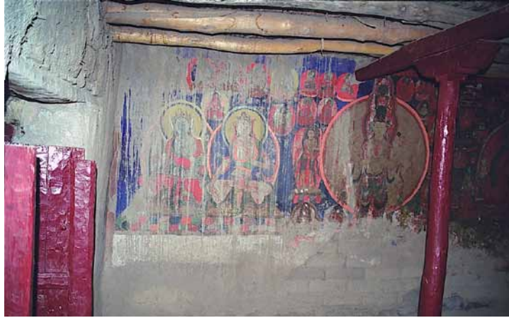
Fig. 450 Interior decoration of the temple room (4), showing the wall paintings on the front area of the southwest wall, which have suffered damage and show signs of later renovation work. Neuwirth 2002.
