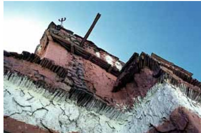
Fig. 574 Right: The periphery of the flat roof is secured with stone slabs. Neuwirth 1998.
