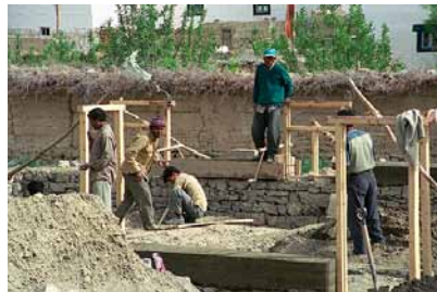
Fig. 556 Left: The lower zone of the exterior wall is built of quarried stones, window frames and door frames are integrated. Neuwirth 2002.
