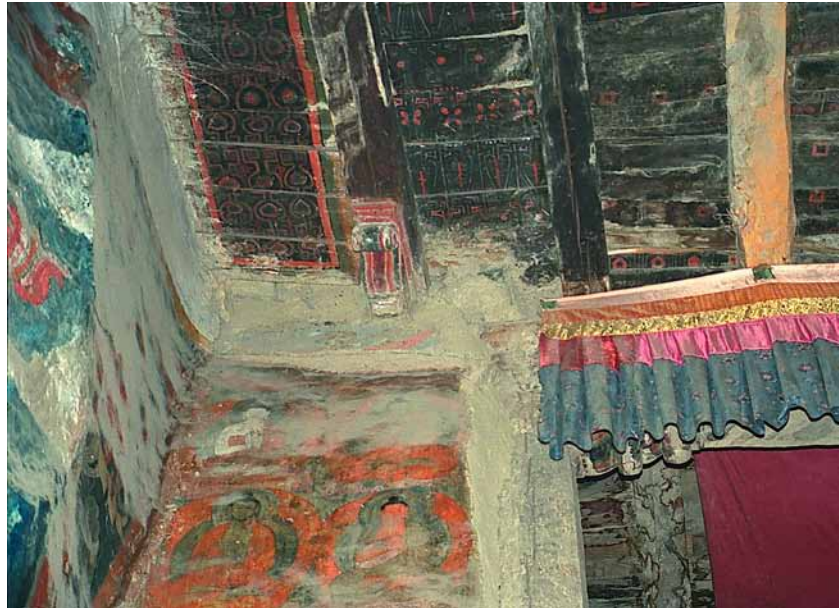
Fig. 412 Change in the ceiling construction from the south part of the west wall to the apse. In the foreground, one recognizes the fracture in the plaster surface of the south wall, the detachment of this surface extends over large parts of the south wall. This surface was later repainted. Neuwirth 2002.
