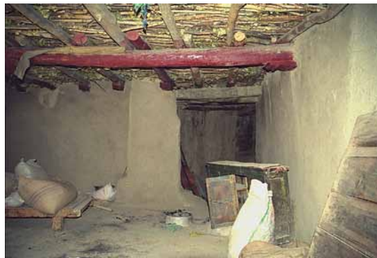
Fig. 275 The south wall in the room above the New Entry Hall. The entrance to the space between the Main Temple and the Large 'Brom-ston Temple is located in the corner. It can only be entered from here. Neuwirth 2002.
