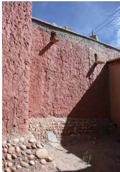
Fig. 562 Right: Securing the ground zone with natural stone walls with cement mortar at the Main Temple of Tabo. The horizontal surface of the base increases the moisture level and destroys the surface of the wall on the inside. Auer 2003.
