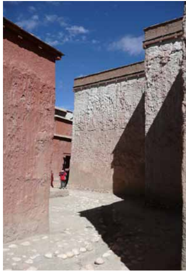
Fig. 40 Overleaf: The southeast elevation of the Main Temple. Below the roof plan of the Main Temple, showing the unroofed corridor between the inner core, the circularly arranged outer chapels, as well as the renewed skylights on the roofs. © Neuwirth & Auer, TU Graz 2020.
