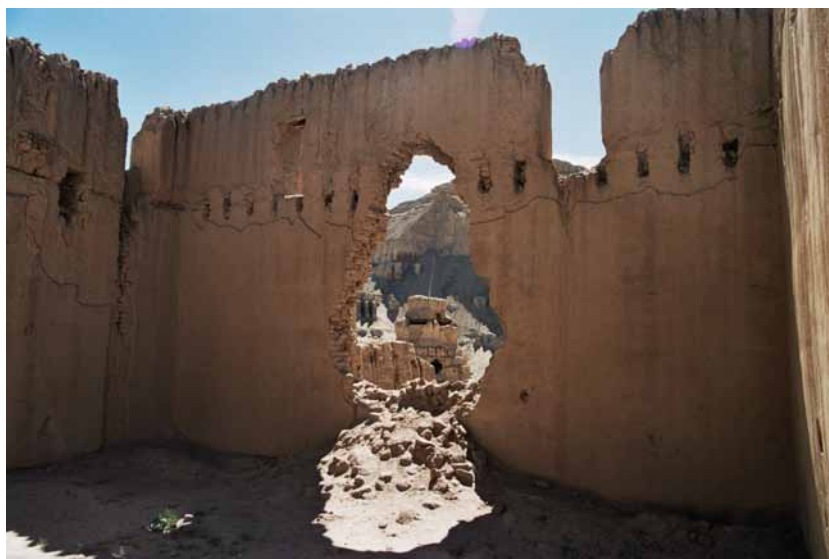
Fig. 136 Interior view of the wall between the entrance area and the main room. The beam holes can be used to reconstruct the former room height and the construction of the ceiling, which has since disappeared. Neuwirth 2007.
