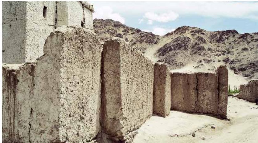
Fig. 563 South wall of the outer circumambulatory of the Main Temple of Nyarma. The cracks at the corners and connection points show the weak point of the wall. The crack in the wall field can be attributed to a settlement of the foundation layer. Neuwirth 2003.
