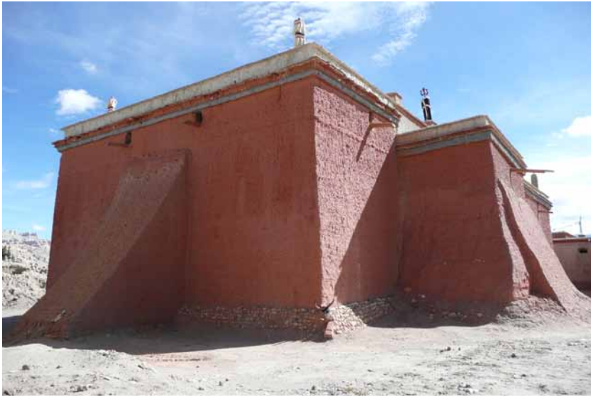
Fig. 87 The wall pillars of the southwest and the southeast façades determine the outer appearance, giving it its curved shape and its size. In the zone above, constructive changes in the rising masonry are visible. The base zone is made of small river stones and surrounds the façades of the entire temple, but was left out in the area of the supporting pillars. Auer 2007.
