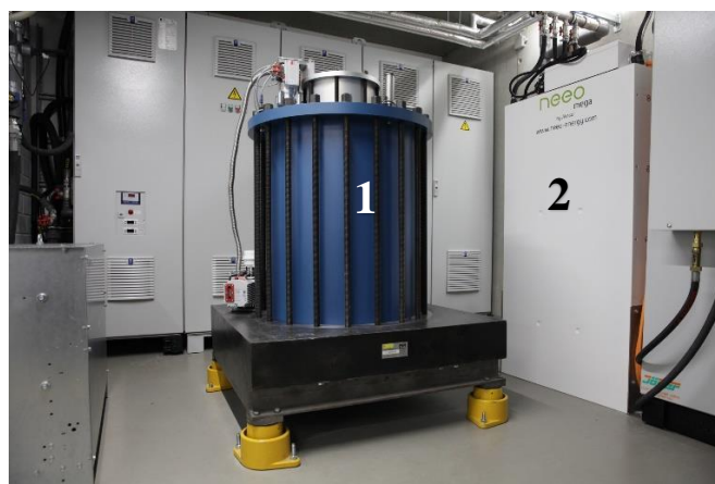
Figure 1: Hybrid Energy Storage System 1: Flywheel, 2: Lithium-ion battery
