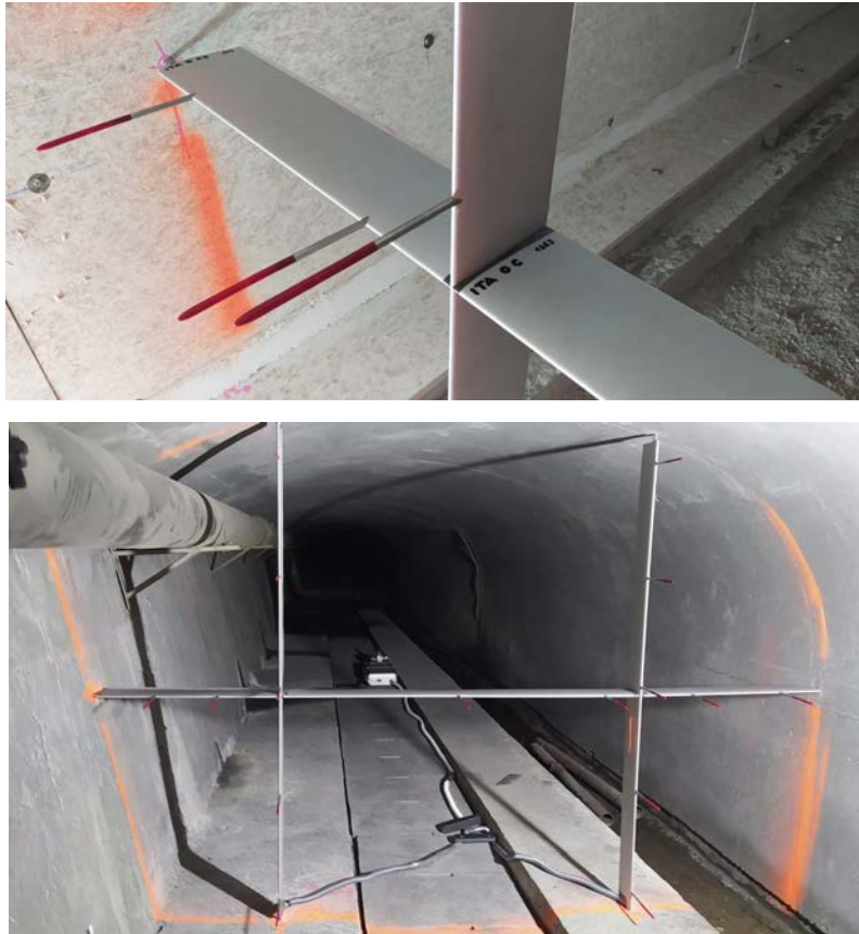
Figure 5: details of the Pitot-probes system (above) and general view (below) as installed on the French side.
