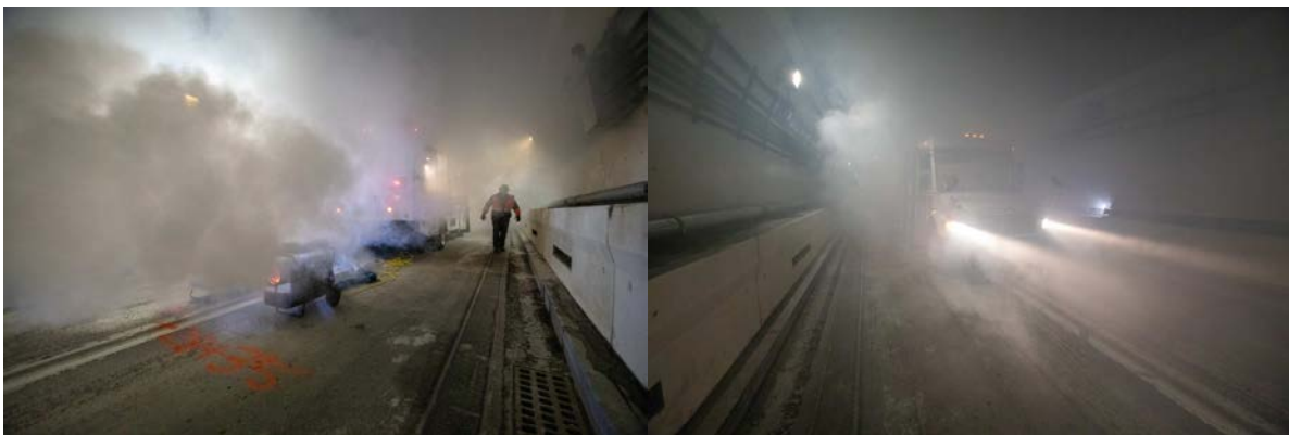
Figure 7: Images of the Delve Stacey Agnew Smoke Bus at various stages of different tests, producing copious quantities of hot ‘smoke’ in service of demonstrating visually the ventilation system performance.
