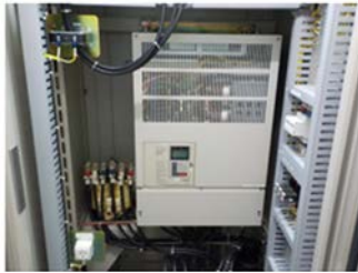
Figure 5: 3-level inverter unit in the control
