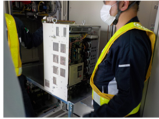
Figure 6: Exchanging the inverter unit
