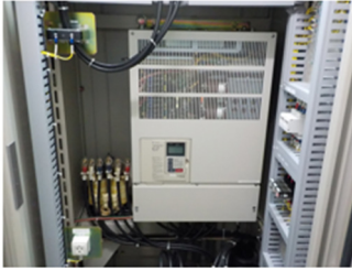
Figure 5: 3-level inverter unit in the control
