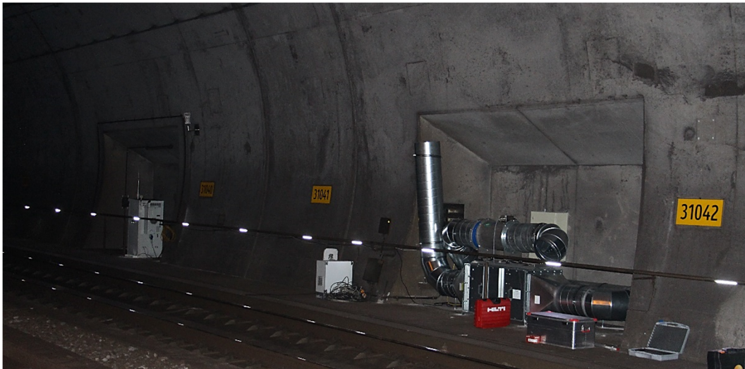
Figure 5: Tunnel Münster - installation of ventilation system including double-stage filter.
