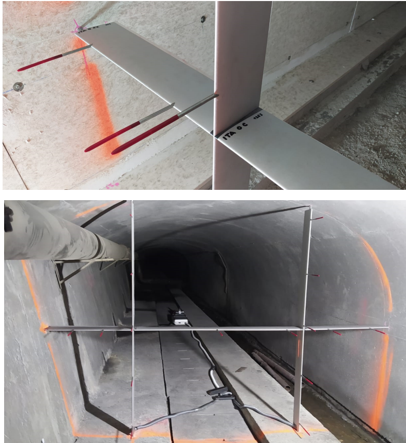
Figure 5: details of the Pitot-probes system (above) and general view (below) as installed on the French side.
