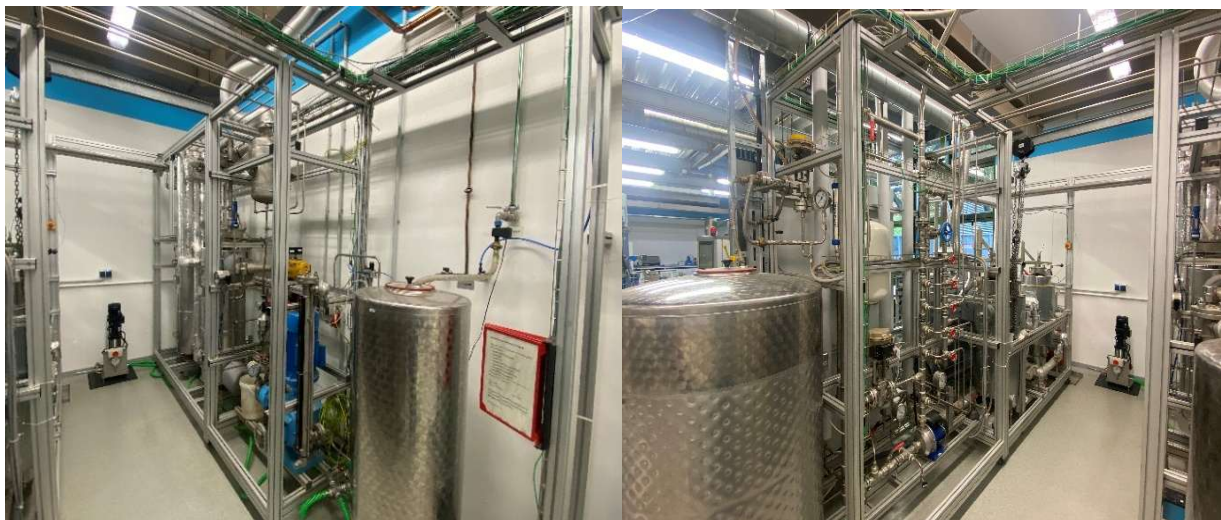
Figure 1: Pretreatment pilot plant for hydrothermal pretreatment
